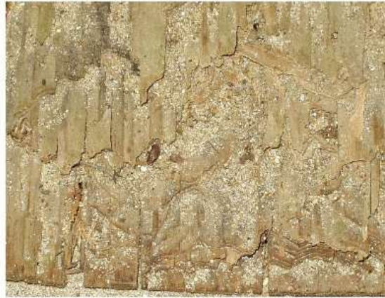
Wood damaged by termites
