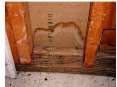
Basement Water Damage
